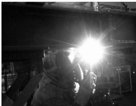
Photo 4.1 Overlay by overhead welding without backing-less process applied the special welding material at the full-size beam-to-column assemblies test production
