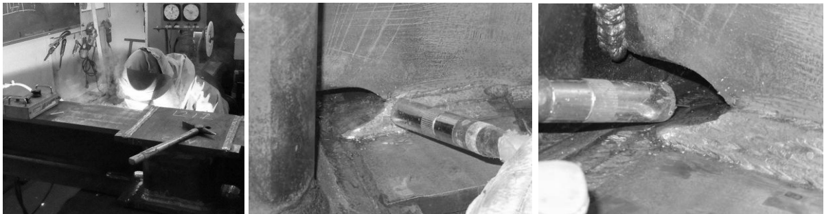
Photo 2.2 Welding situation and welding torch position at the tip of overlay welding in the scallop
